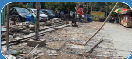
The civil work after whitewashing is hindering progress.
